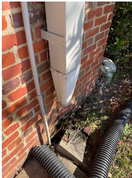
Downspouts draining directly against building foundation with evidence of damage to surrounding soil
