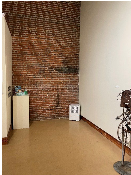
In-gallery dehumidifer under evidence of past water penetrations
